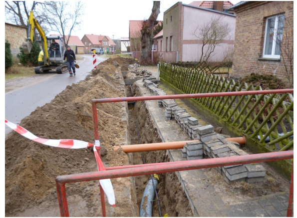
Figure 14: District heating with biogas energy improves efficiency and can be a bonus for rural infrastructure. Photo: N. Hölzer, MEP.
