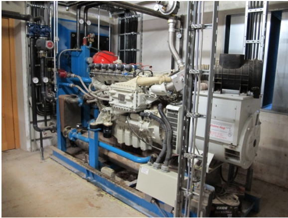
Figure 29: CHP: Biogas for Electricity and Heat. Photo: V. Jaensch, RENAC.
