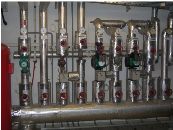
Figure 23: Heat distribution in biogas plant. Professional concepts may utilise a large proportion of heat produced. Photo: MEP.
